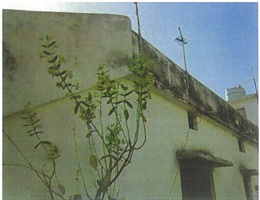
Mark flat projections of chhajas; above smaller & larger windows. Both projections have gathered moss (blackening effect is apparent) only redeeming feature is that the projections by themselves have allowed the rest of the fascia to be without any effect.
